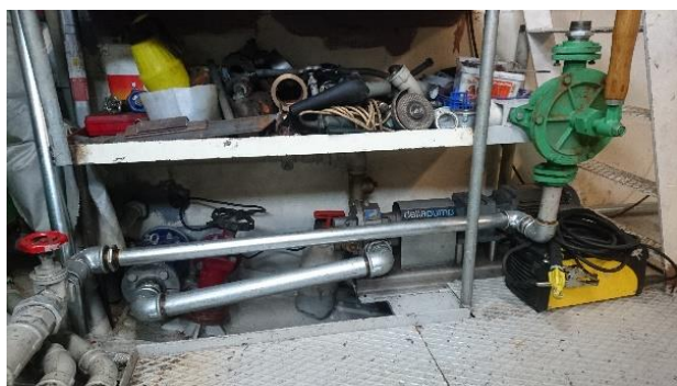
Nikkepumpe for lensing. Brannpumpe under.
