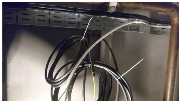
El-kabling i casingen
